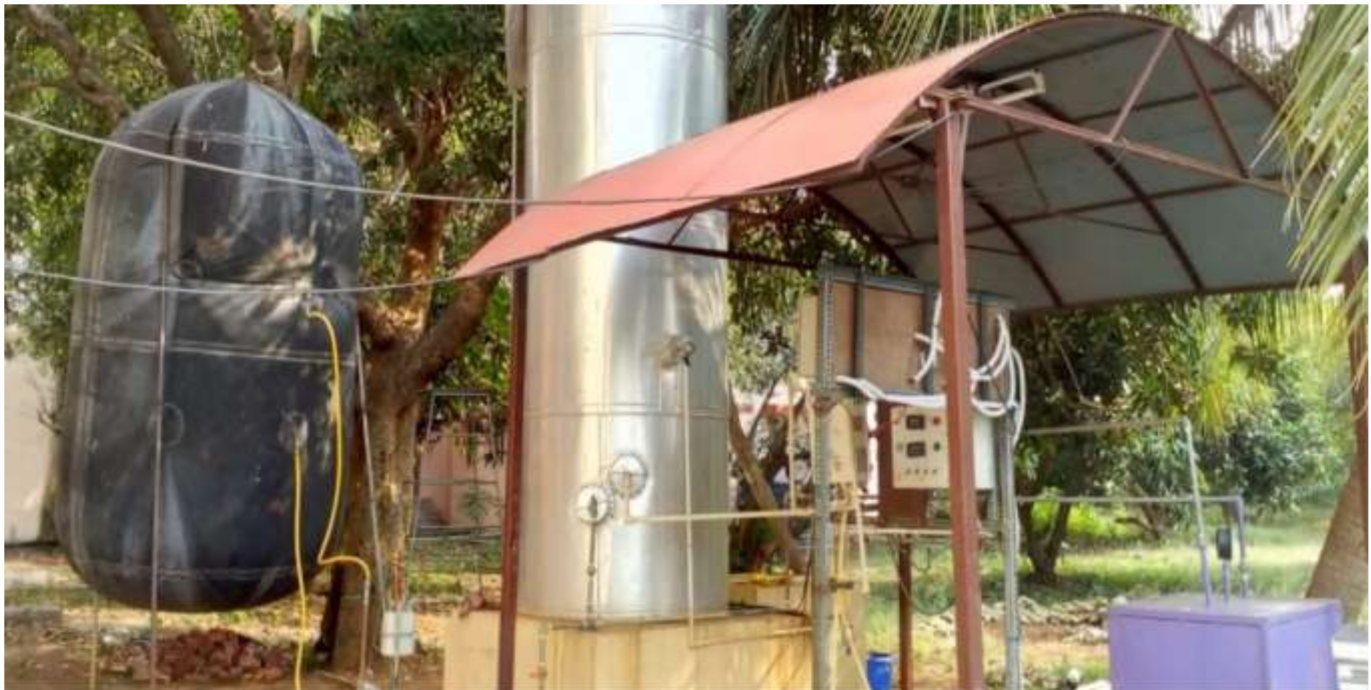
FIG: Biogas Plat at MVGR College of Engineering
