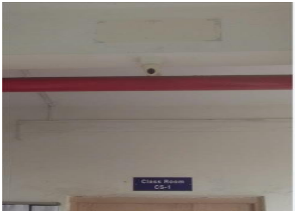
Camera on class room entrance
