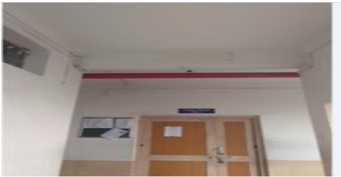
Camera on class room entrance
